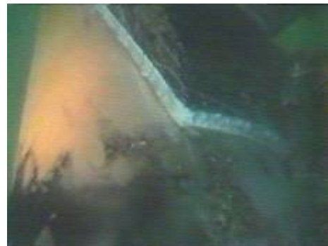
Photo shows underside of weld repair
