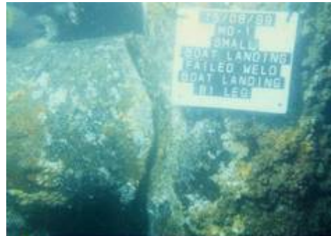
Photo shows the failed weld/ member
